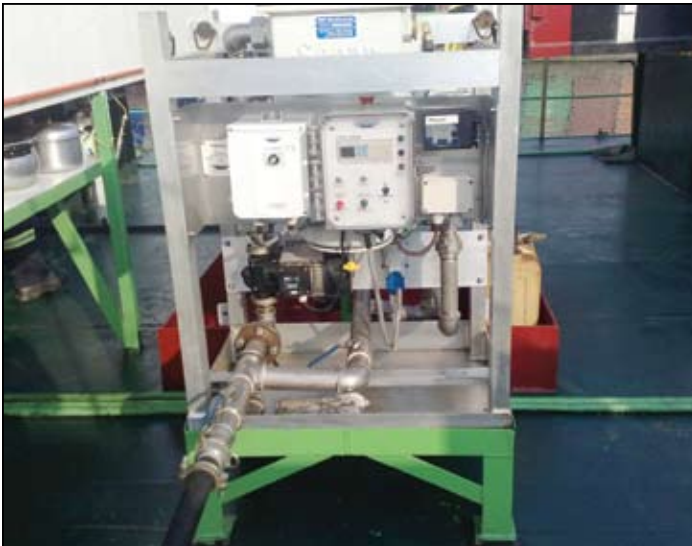
Fuel Polishing System installed on dredging barge.
