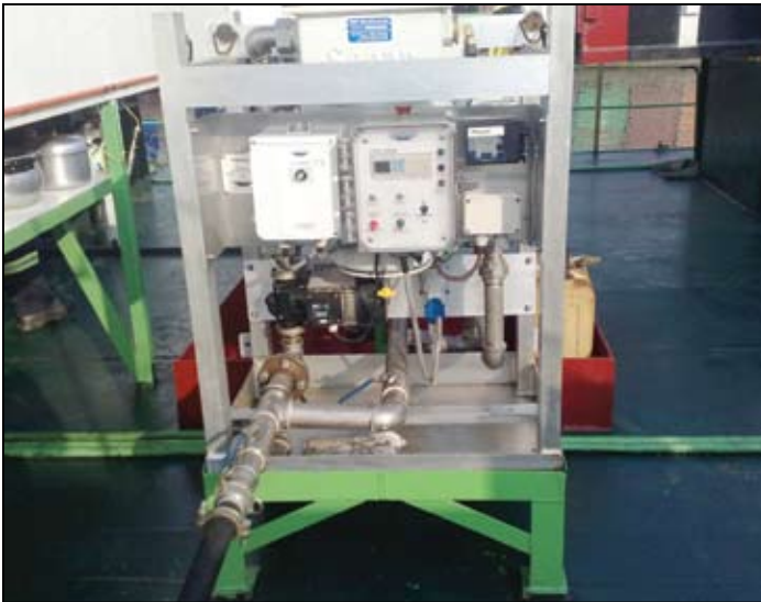
Fuel Polishing System installed on dredging barge.
